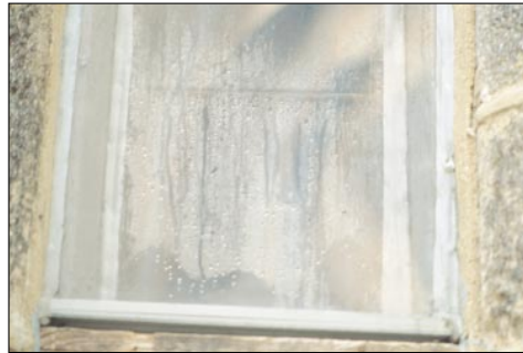
Rigid coverings on stained glass not only save minimal heating energy but can trap heat and moisture, which ruin the window and its frame. Photo by Jean Farnsworth
