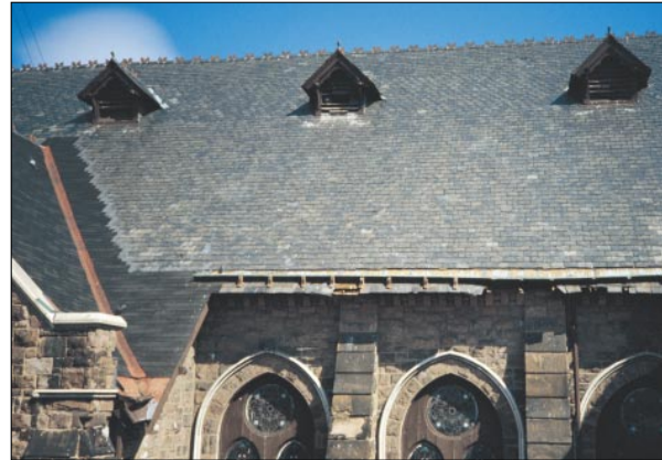
Dormer vents provide natural ventilation for this church. Overnight summer cooling reduces air conditioning loads.
